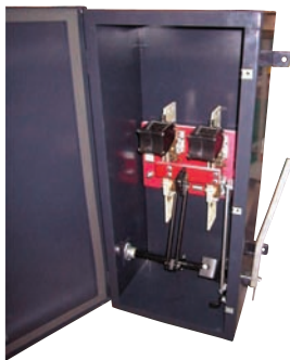
Mill Switch (PMS)
